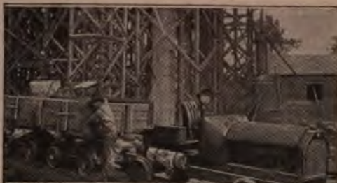
An Old Six-Cylinder Touring Car was Cut Down by a Construction Gang to Act as a Narrow-Gauge Locomotive, and Haul Building Material
